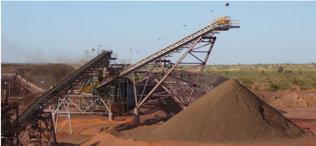
New surge bin in operation
