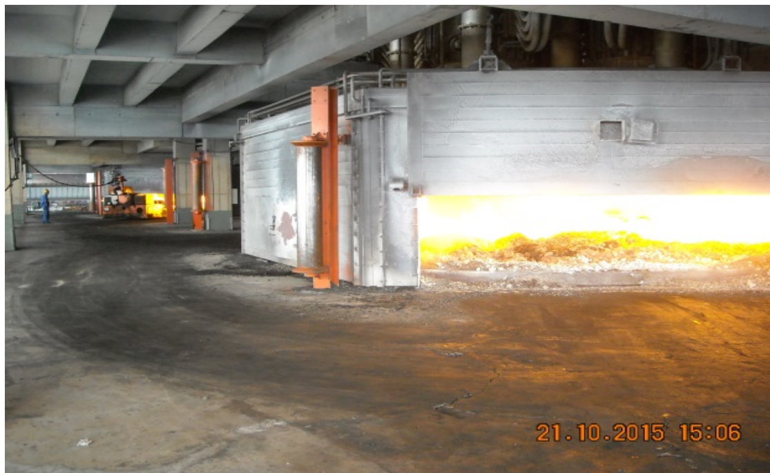
B01 Furnace at work
